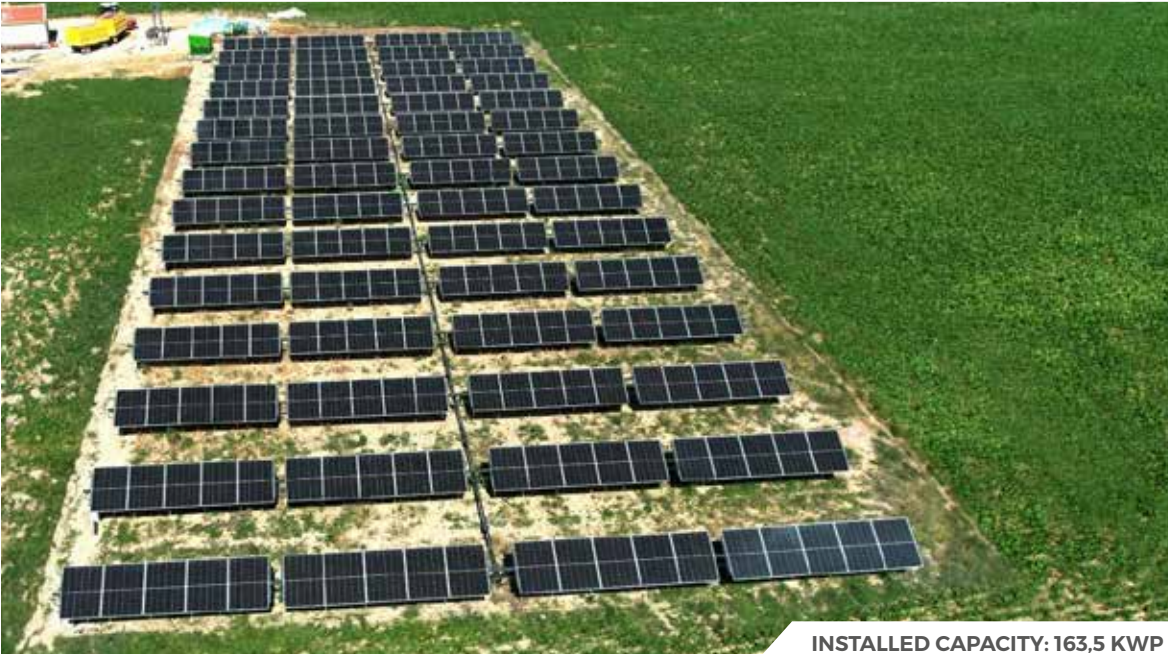
INSTALLED CAPACITY: 163,5 KWP
